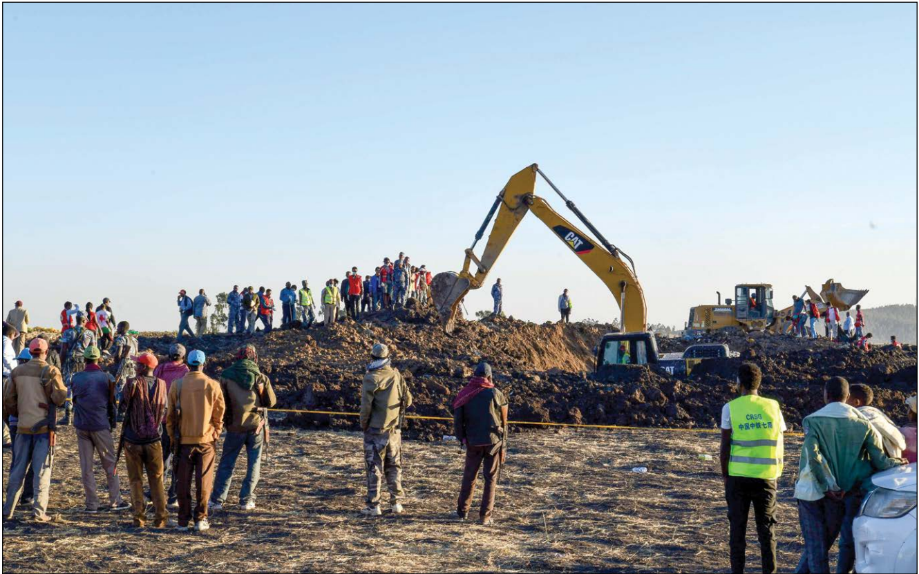
Tractors excavate the scene of the Ethiopian Airlines Flight ET 302 plane crash, near the town of Bishoftu, southeast of Addis Ababa, Ethiopia, 10 March 2019.
